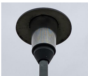
Faulty lanterns to be replaced with new LED models
